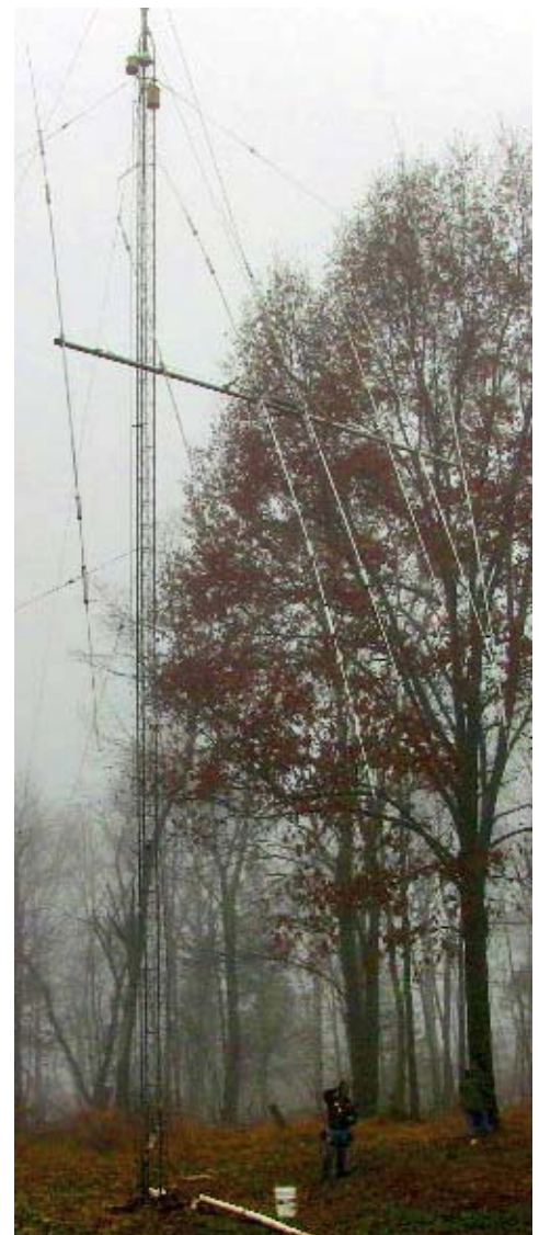
Mosley Pro-67-C is lifted up Bill's tower. This giant antenna covers all seven amateur bands from 40 to 10 meters.
