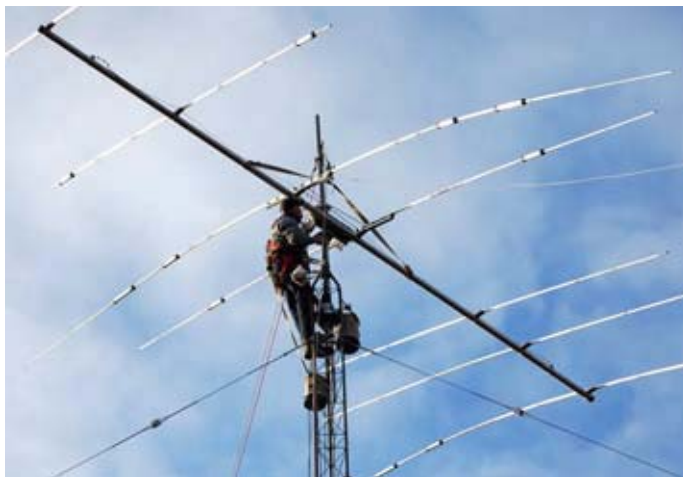
Mosley antenna is mounted on the tower by Ray W2RE. [Photos by N2KZ]
